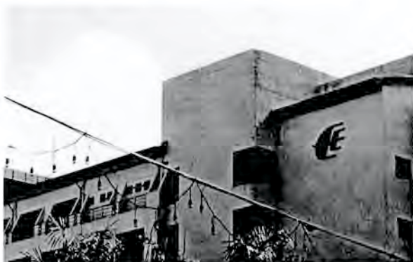
Figure 2. The same building photographed some years later showing the stricken point (top right).
