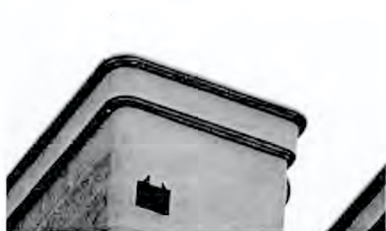
Figure 4. The same building photographed six months later showing two (out of five) new stricken points.
