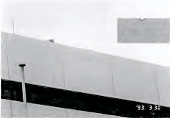
Figure 9. A stricken point on the straight edge of the roof (far right). Inset: A close up of the stricken point.
