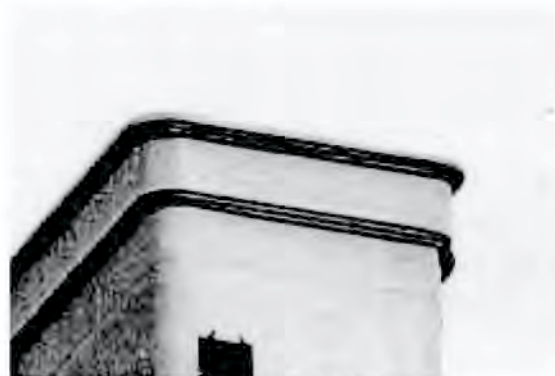
Figure 3. A photograph of the Villa Putra apartment taken in February 1999 showing the undamaged upper level roof. Two stricken points had been observed on two other lower level roofs.
