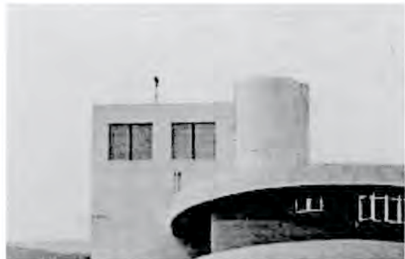
Figure 8. A stricken point located on the curved portion of the roof (right) with an undamaged sharp corner nearby (left).
