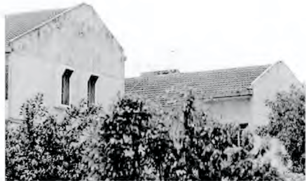
Figure 7. Two adjacent residential apartments with similar stricken points on the roofs.
