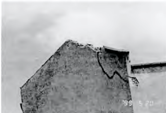
Figure 6. A close-up photograph of a severely damaged façade of a commercial building. In this case, the stricken point appears to be on the slant side of the façade instead of on the pinnacle.
